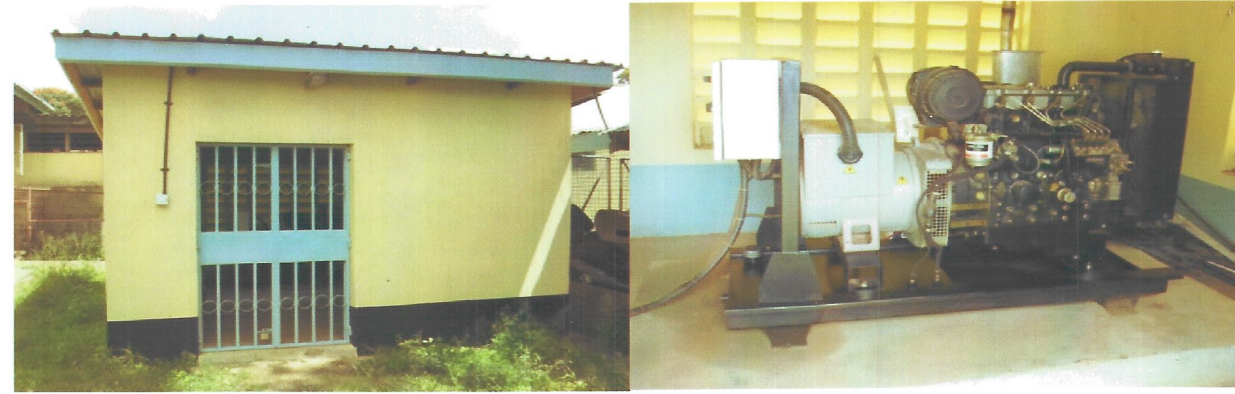
Automatic backup Generator - 2006
