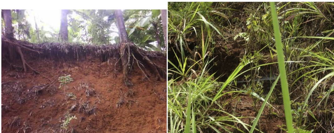
(g) Thick soil layers with roots only holding the top soil layers (h) inappropriate vegetation on already developing cracks
